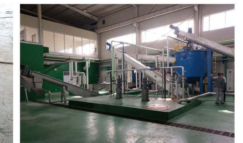
Kitchen Waste Treatment System
