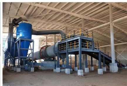
Drying System Equipment
